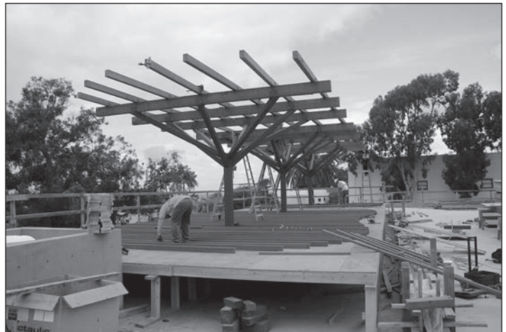
The steel and ipe wood trellis under construction at the northwest corner of the plaza deck currently designated at the Pacific View Terrace. The final top layer of 2 x 4 ipe boards are laid out on the floor, and will mimic the organic structure of three threes when installed.
