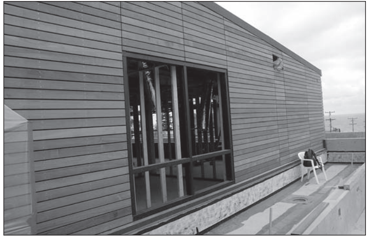
The view of the north wall of City Hall looking west shows the ipe wood siding. Ipe is a dense, renewable wood that is extremely durable, and is being used in many exposed elements to withstand the impacts of the coastal environment.
