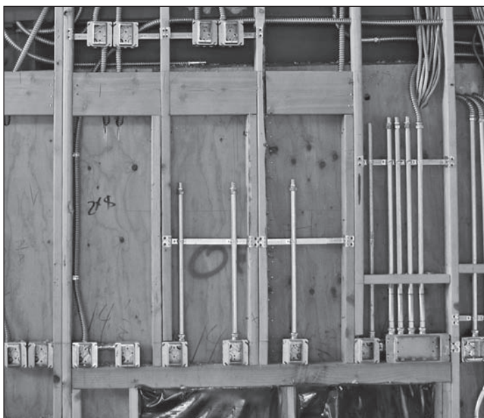
Twelve switch boxes in a row along south wall of Town Hall.
