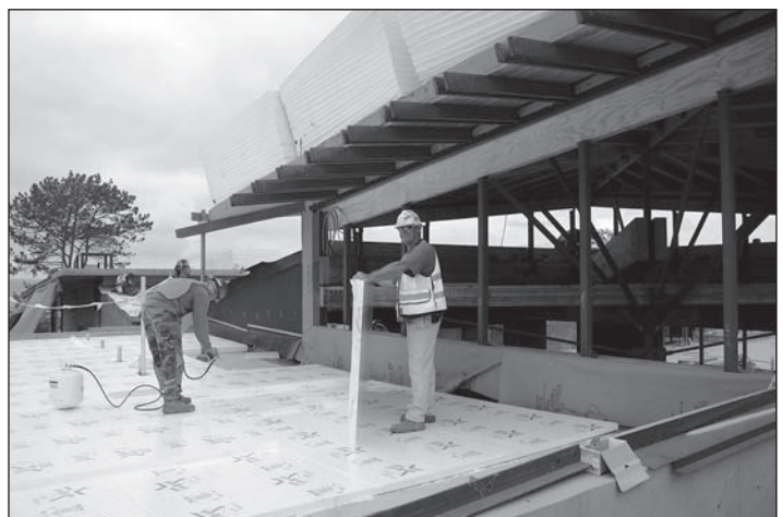
Construction workers installed two layers of foam insulation over the roof of the TV studio just south of the new Town Hall. Photos Don Mosier. □
